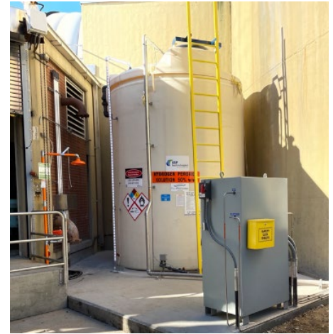
Peroxide Holding Tank
