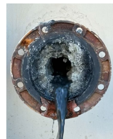
Centrate Tank Drain
